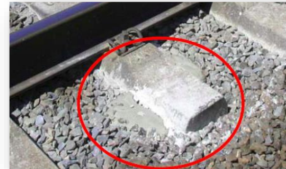
Deterioration of Sleeper and Ballast
