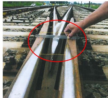
Deterioration/Settling Crossing Nose
