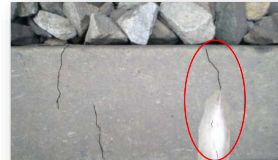
Cracks in Concrete Bearers
